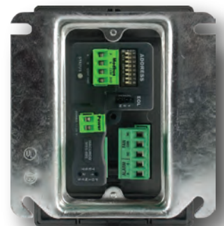
Installed MRS-485 View
